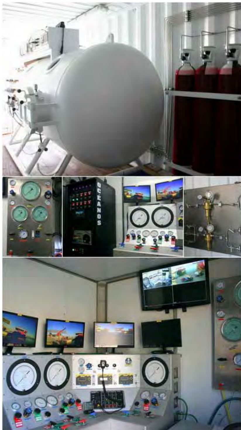
The new dive control station
